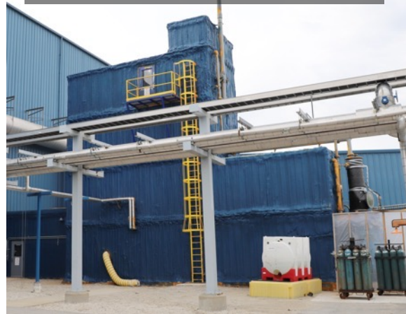
Molten Salt Purification Plant Elmore, OH
