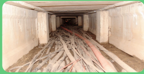
Low and Medium Voltage Cable Aging Management
